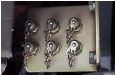
Hydraulic pressure check points The pressure test points are grouped together. (Main pressure, steering, braking etc).
